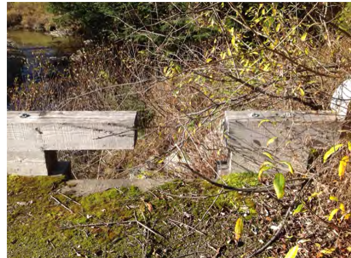
missing section of guardrail
